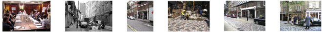
Above, left to right: Stakeholders consultation on Monmouth Street with Camden officers; Monmouth Street in the 1960s; Before works; Laying multi-coloured (flat) setts; The works completed in 2006; Being admired by Princess Anne.
